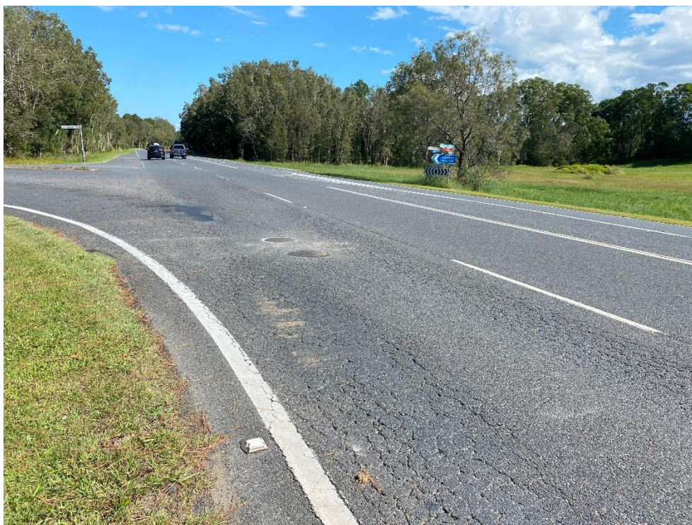
Looking south along Hogbin Drive at the existing intersection. Crocodile cracking and minor rutting is present within the wheelpaths of the southbound slow lane.
