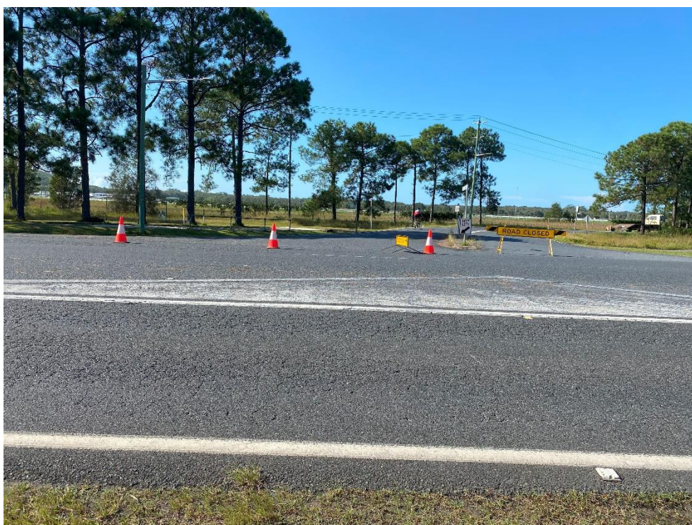
Looking east across Hogbin Drive at the existing intersection with De Haviland Way. Crocodile cracking and minor rutting is present within the wheel paths within Hogbin Drive.
