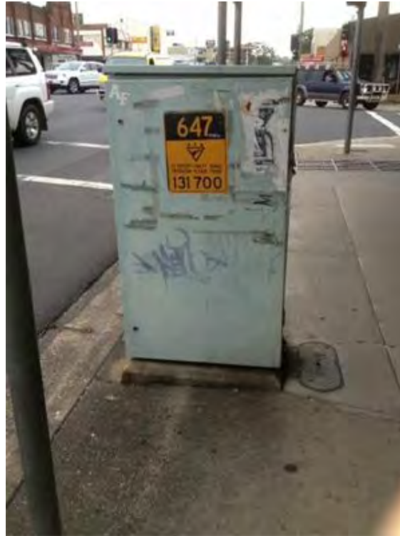
Traffic Signal Box - intersection of Pacific Highway and Harbour Drive
